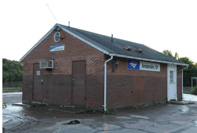
High water mark on the Amsterdam station
